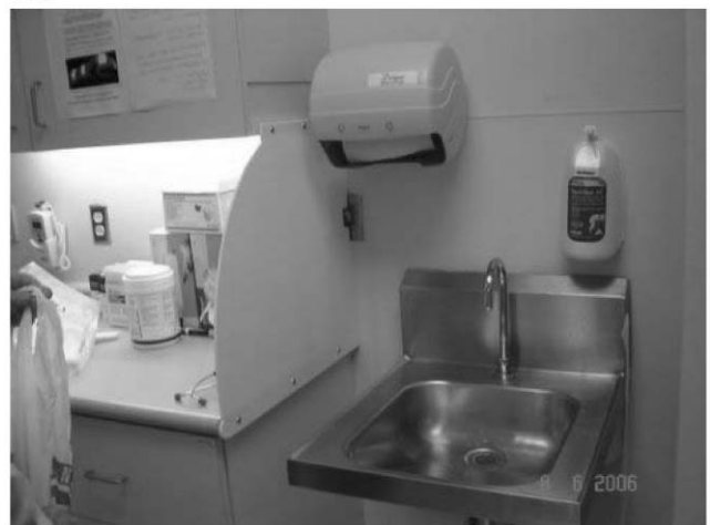
FIGURE 5. Sink and counter design in the medical/surgical intensive care unit where the outbreak occurred. Panel A, before renovation; panel B, after renovation.
